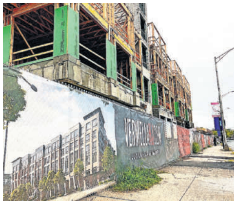
The Vermella Broad Street project will add 296 apartments to Newark’s Lower Broad Street neighborhood. Steve Strunsky, for The Star-Ledger
